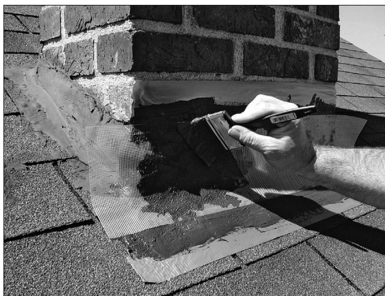
This patch system repairs and seals the flashing around the base of the chimney. A piece of mesh is covered with a tough polymer material that adheres well.
