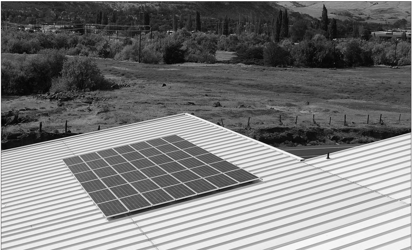
Solar panels on the roof of the PUD garage generate electricity that is used at the facility.
